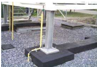
Container Grounding System
