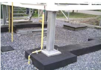
Container Grounding System
